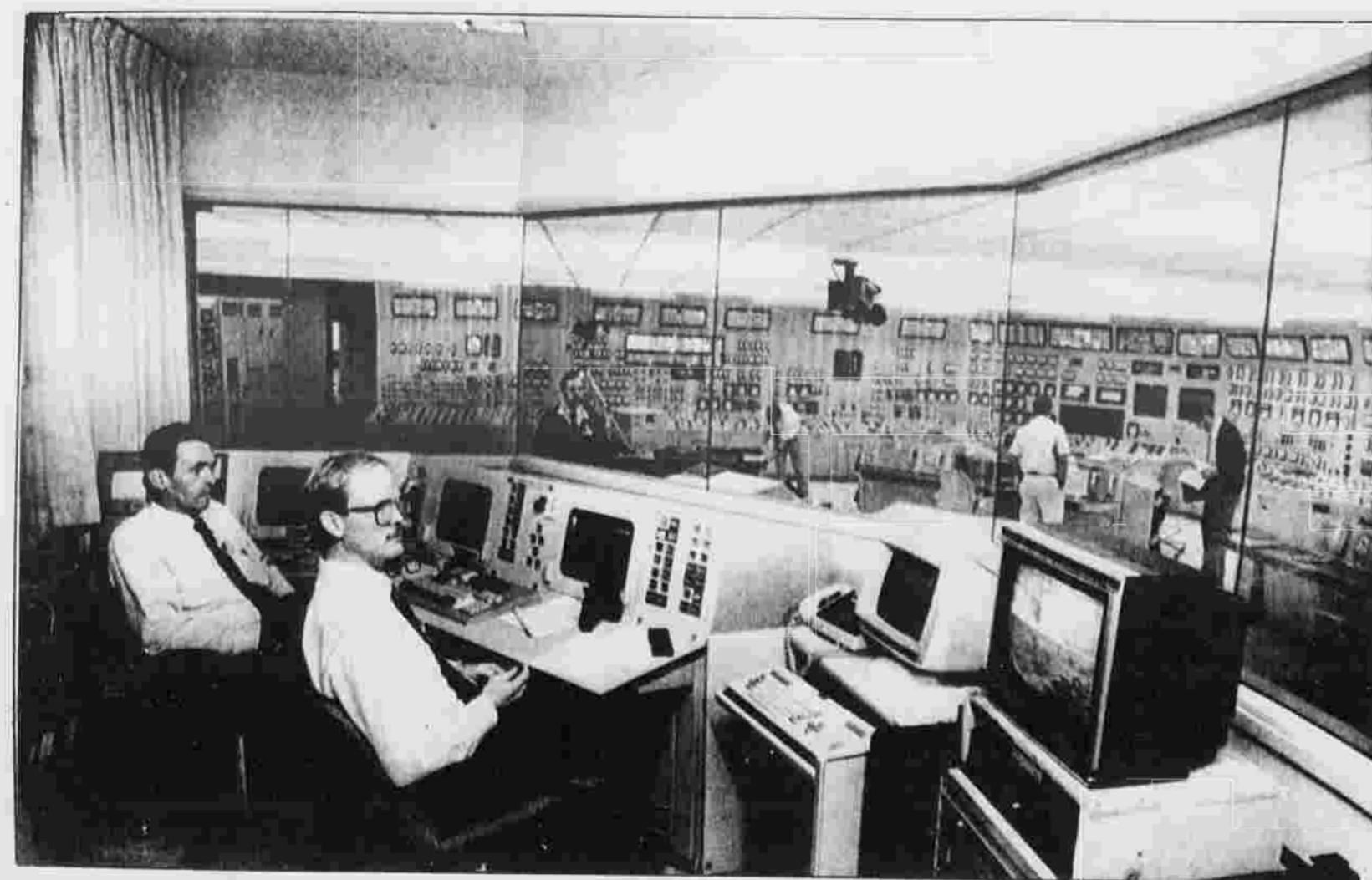
READY FOR TESTING — Millstone III nuclear power plant instruction operators Larry Allen, left, and Charles Ryan sit by their consoles in Waterford Wednesday as they prepare nuclear disaster tests. The simulated control room is an exact duplicate of the Millstone III control room. Last week, six of the 12 operators at Millstone III flunked requalification tests.
